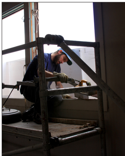
Ben Isaacson of Vintage Window Restoration, LLC uses infrared light to remove old paint from a window in the mezzanine of the Armory.
